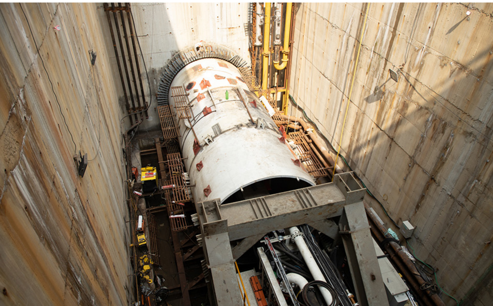
TERRATEC 3.85m diameter Rock Slurry TBM is making strides in Mumbai Sewage Disposal Project-Stage II, PST-1 in India.
