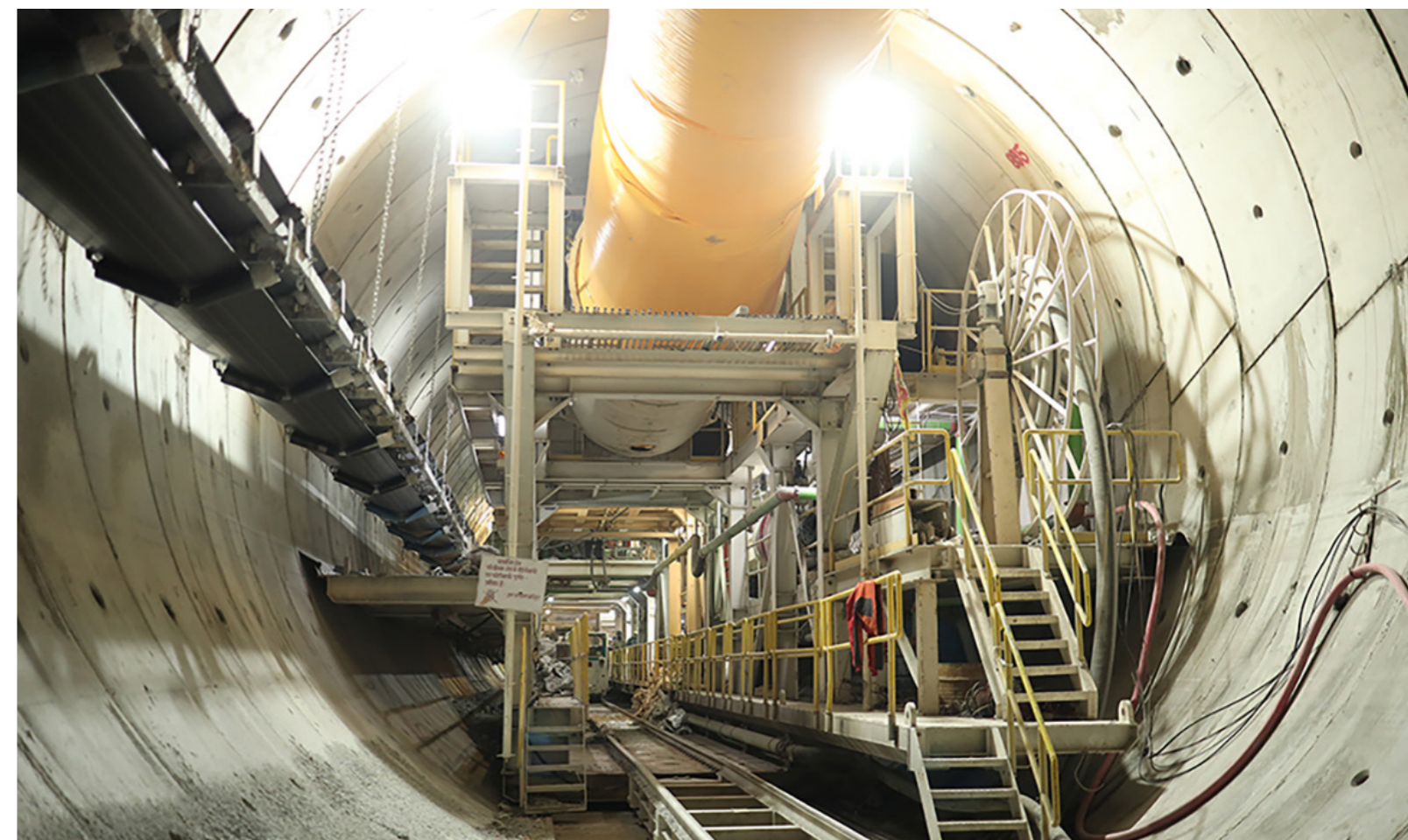
TERRATEC's Hard Rock Double Shield TBM is making great progress for the Vishnugad-Pipalkoti Hydropower project.
